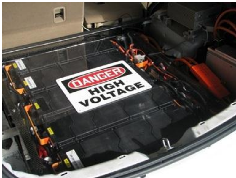
Figure 6.1 A123 battery pack on vehicle
